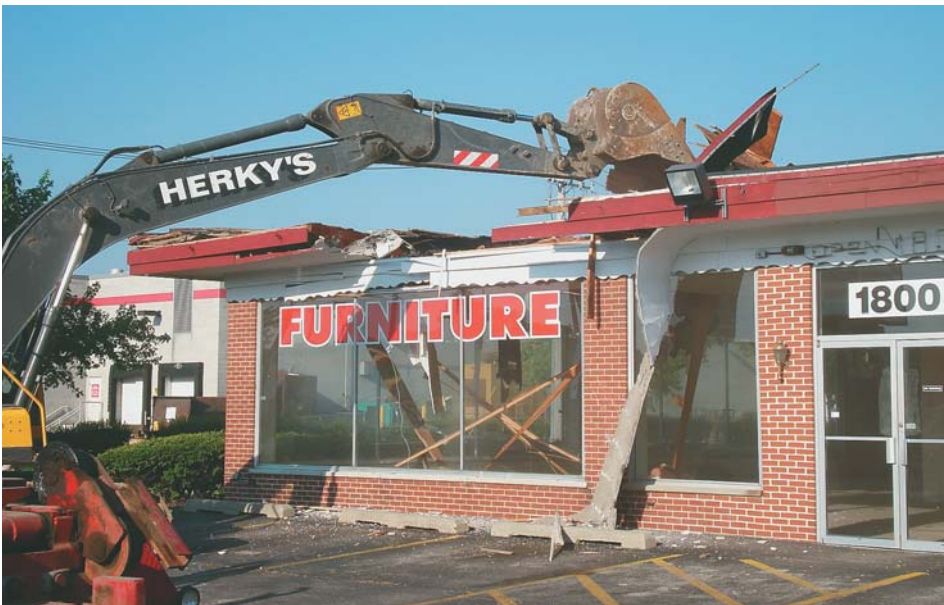
An old furniture and appliance store is demolished before site construction begins.
